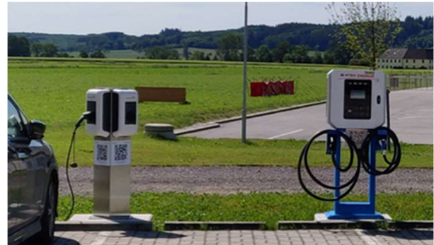
© BEST, Charging infrastructure at the Microgrid Lab.
