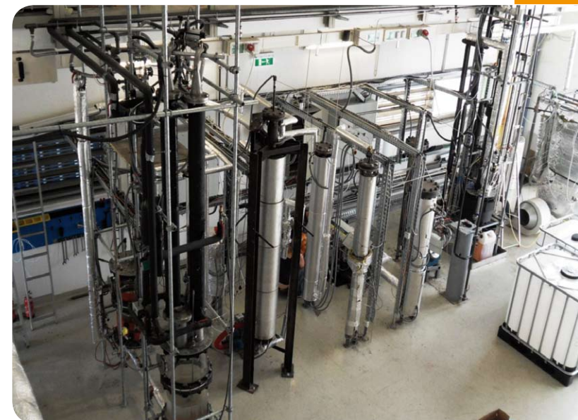
Fischer-Tropsch laboratory facility with gas scrubbing: The synthesis gas is converted to FT diesel in the catalyst filled slurry reactor at temperatures between 200 and 300 °C and at pressures from 20 to 30 bar. Figure: Compression (left), FT reactor (centre), product separation (right)
